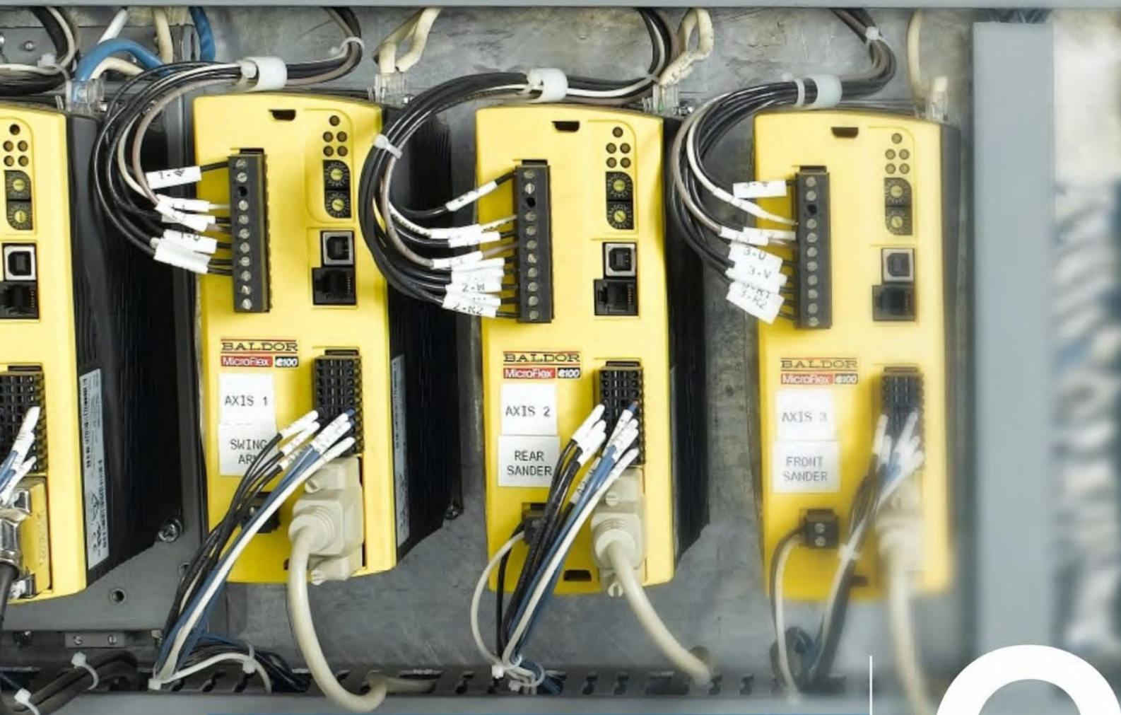
Instrument & Control Cables
